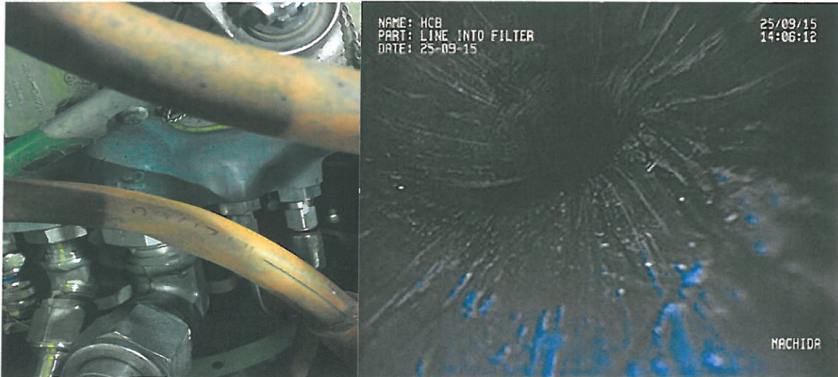
Fig 6: Hose P/N: 70-079H000Y150 KINK ON LINE AND BORESCOPE VIEW
